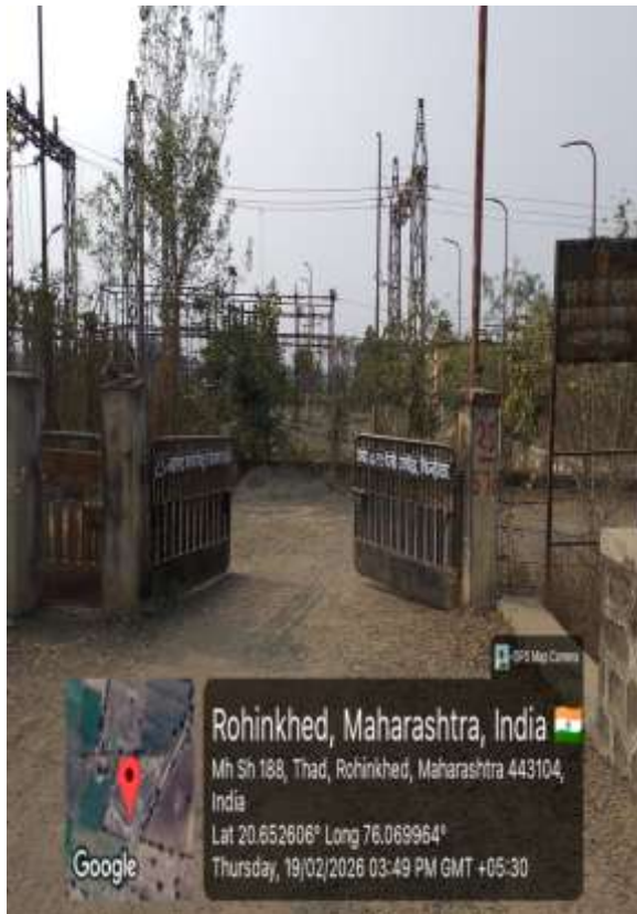
Fig c. Substation at Rohinkhed, maharashtra
