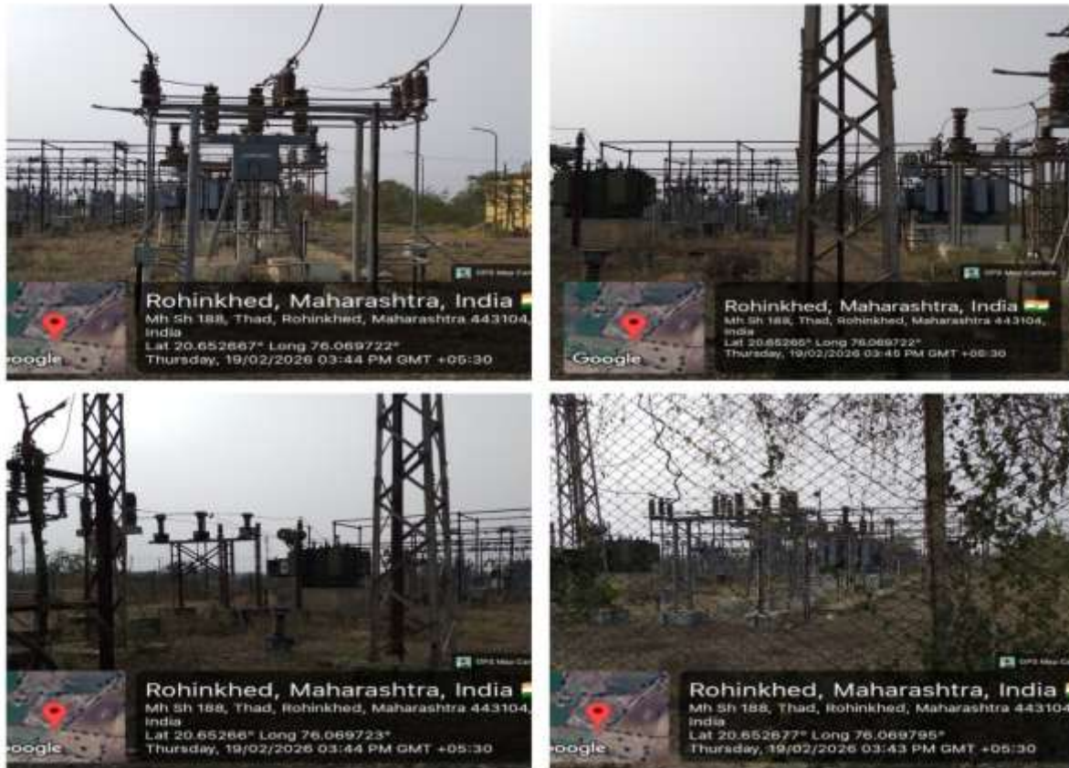
Fig 4.10. Case of 33/11 kV substation located at rohinkhed
